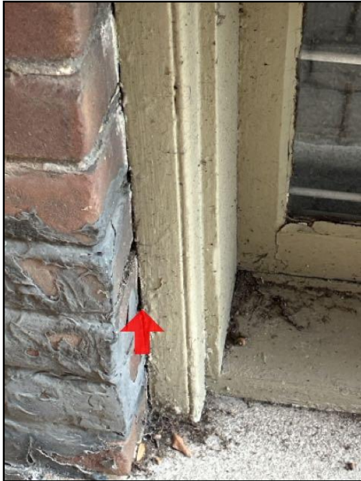
Caulking missing, loose or deteriorated
