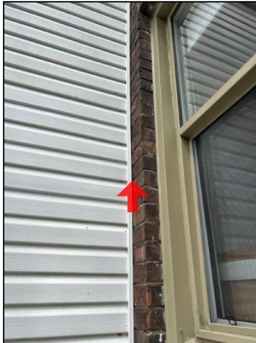
Caulking missing or ineffective
