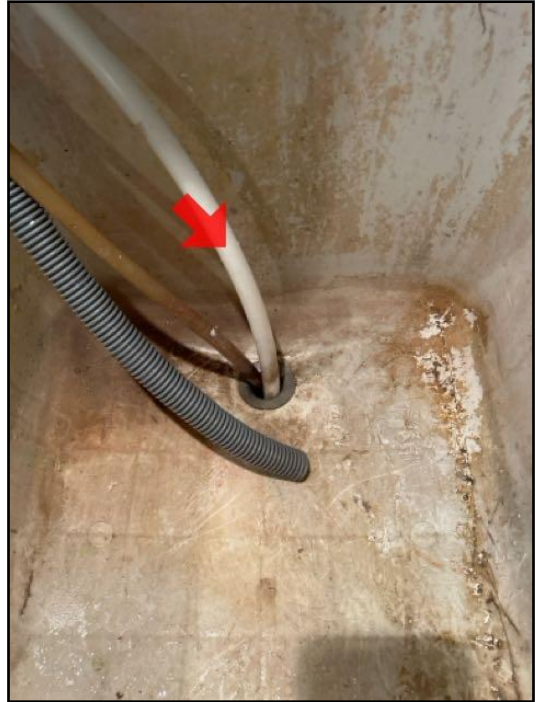
Water filter relief line
