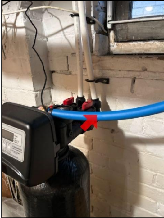
Water filter relief line
