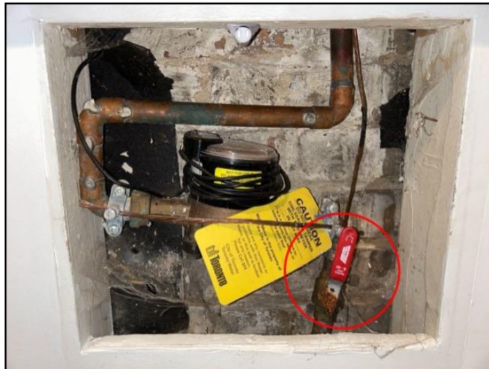
Water shut-off valve
