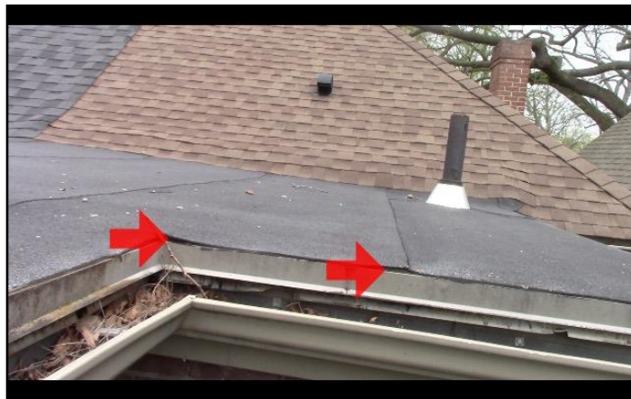
Openings at seams or flashings
