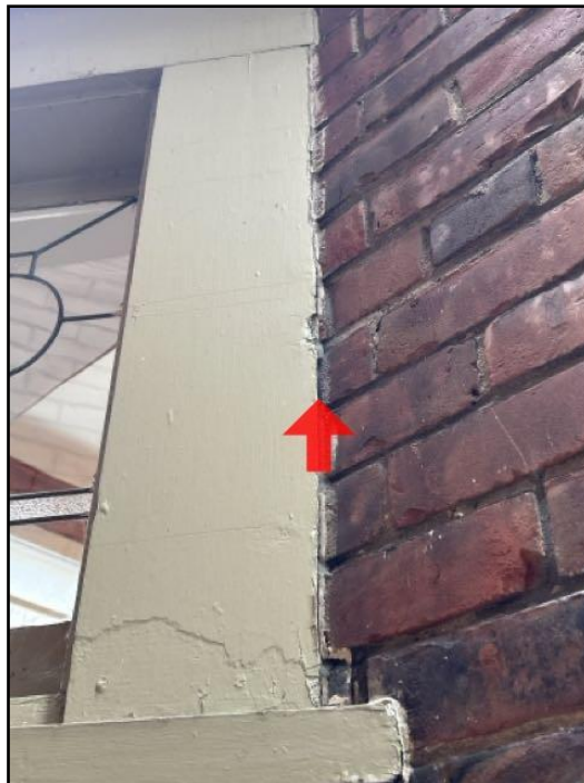
Caulking missing, loose or deteriorated
